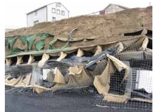
Failed Wainwright gabion wall
